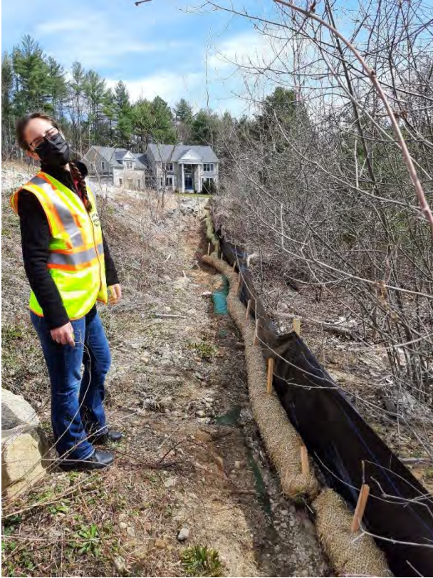
Anna Rogers, Environmental and Inspectional Services Coordinator, inspects erosion and sedimentation controls at a residential construction Site.
