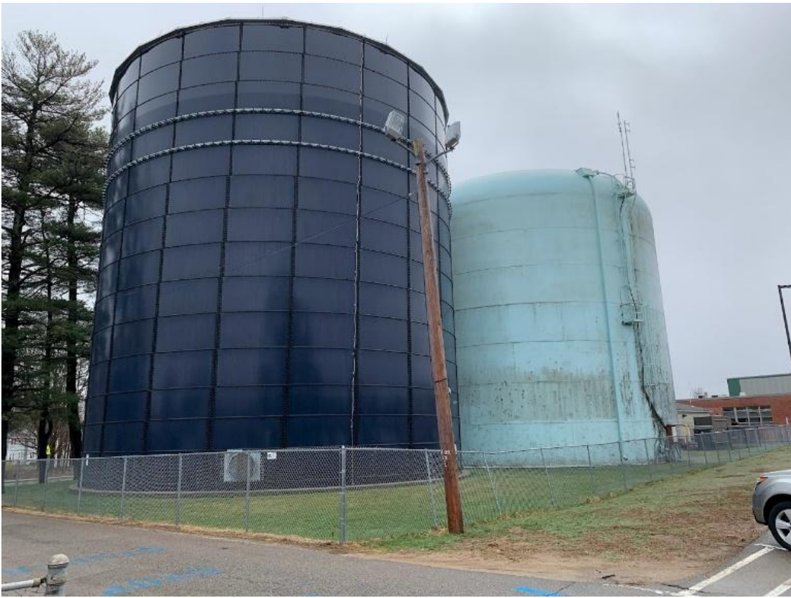
Photo: Water tank that needs to be replaced is the light blue tank in the background. New (2017) water tank in foreground.
