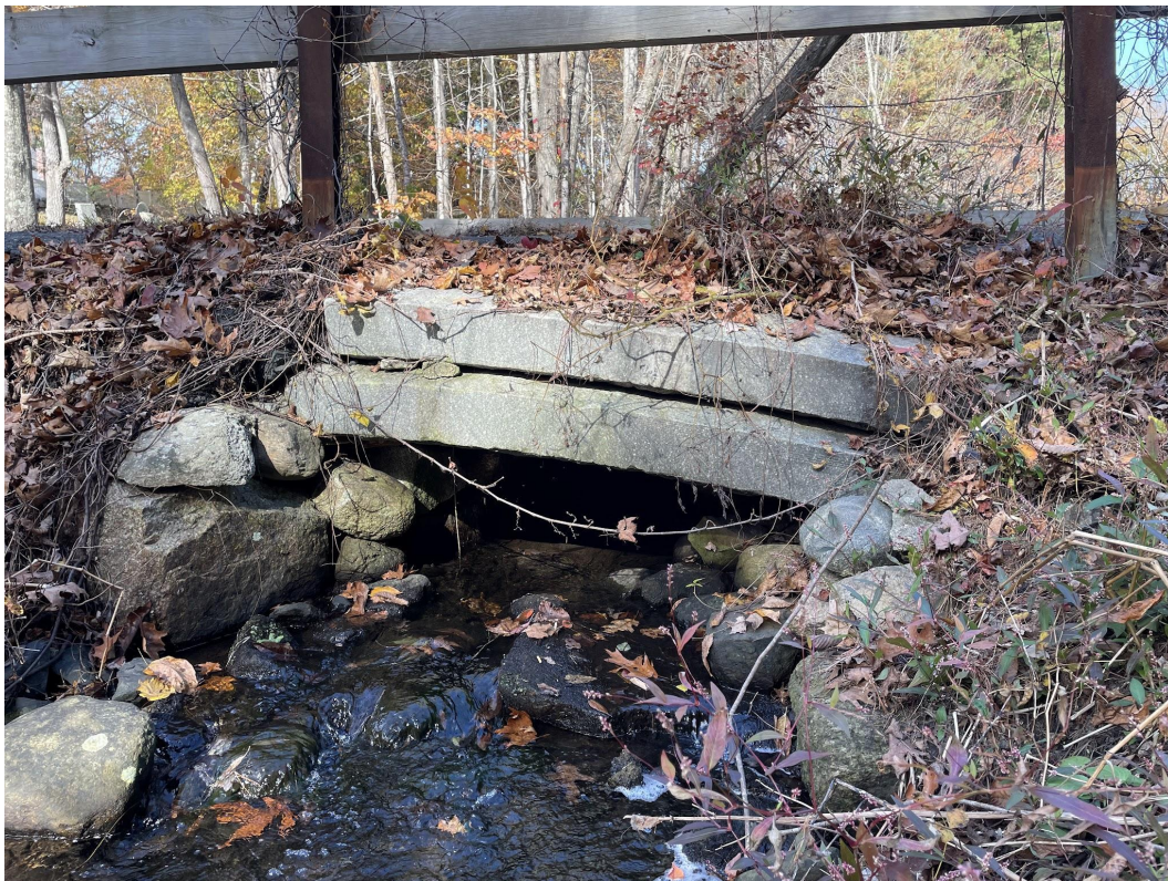
Photo 1: Granite Street culvert, on north side of Granite Street looking south. Town cemetery is located to the right of this photo.
