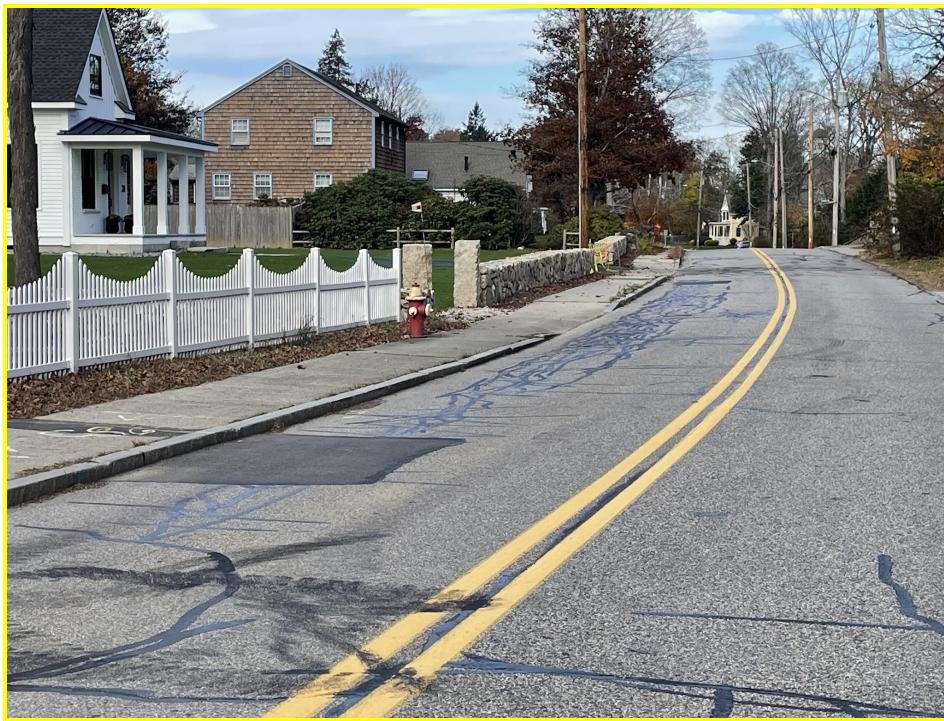
Photo: View looking north on Ash Street. Property at 28 Ash Street is located to the left. Note alligator cracking in the front of the driveway and fire hydrant where ponding usually occurs. Photo taken Oct 27, 2023..
