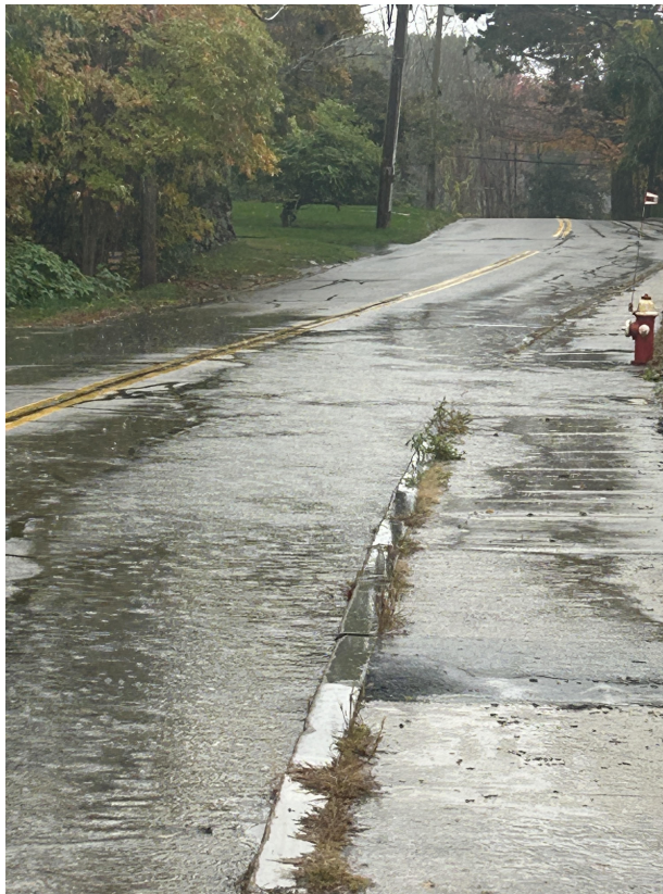
Photo: View looking south on Ash Street. Ponding on road and overtopping of sidewalk during storm event on Oct 21, 2023 from approximately 1 inch of rain. Photo provided by property owner at 28 Ash Street.
